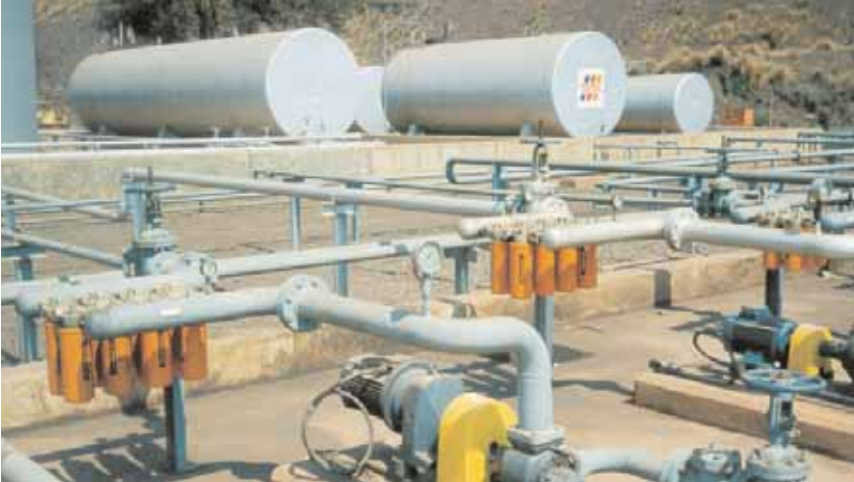
Donaldson Duramax units at this South Africa ore mine filter bulk oil as it runs from storage tanks to delivery trucks for transport to the customer. This parallel filter configuration provides for high flow rates.
