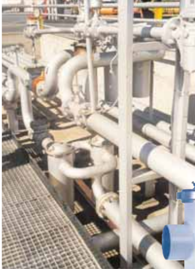
At this oil depot, high-flow/low-pressure HEK11 filters are used to remove both ingressed & induced contamination from oil that is piped around from reservoir to tank.
